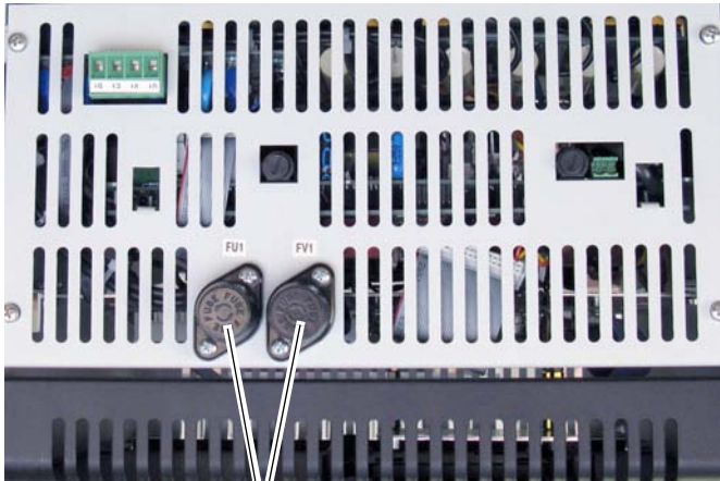
Field circuit fuses
