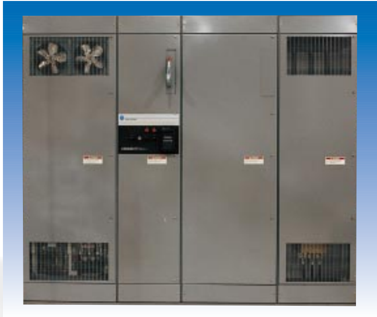
500 HP 1336 PLUS NEMA Type 1 Configured Drive with SMC Style Bypass. (See page 7 for internal view.)
