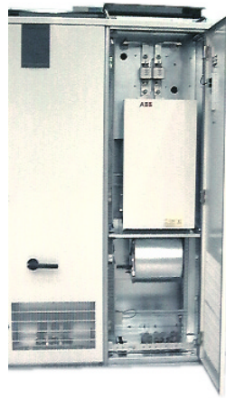
Figure 3-1 A 320 kVA / 500 V drive section
